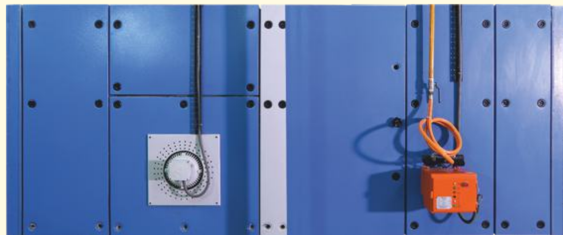
View of Burner Mounting in Chamber
